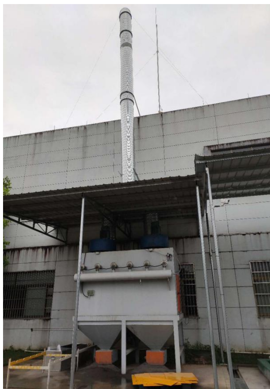
滤芯除尘器+15m排气筒
